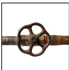
Leaking valves and fittings
